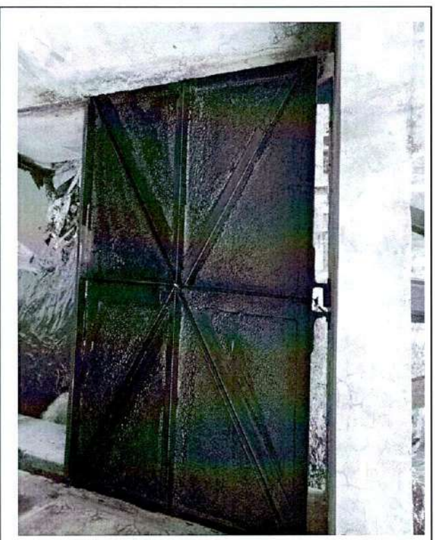
HALISAHAR DRAIN LOCKGATE
